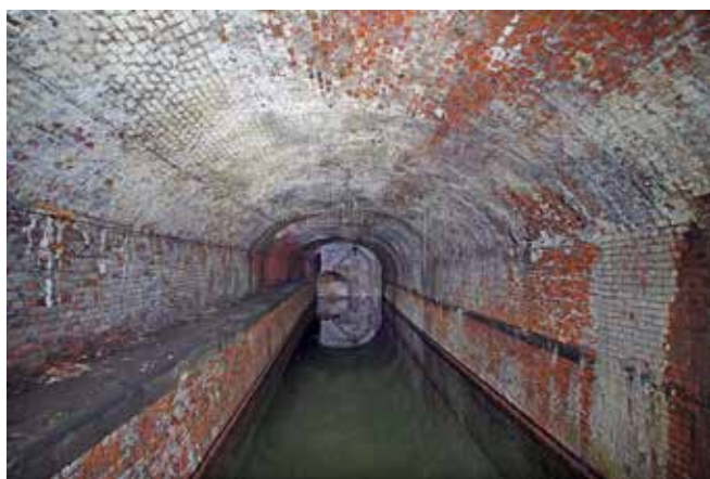
The first main section at the Grape Street end, with the remains of the structure to keep out the damp and cold in the shelter clearly seen on the back wall. Photo Nick Catford
